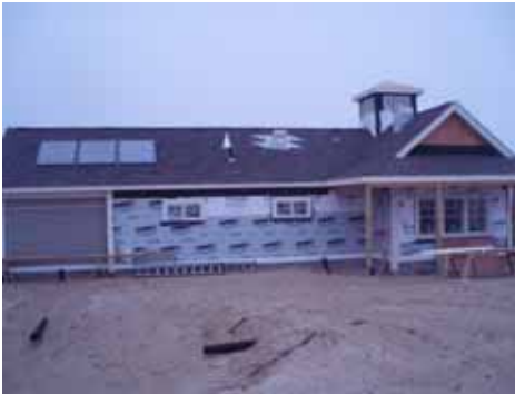
East Side of the Bathhouse – Note the solar hot water panels on the roof which will allow hot water for outdoor showers.
